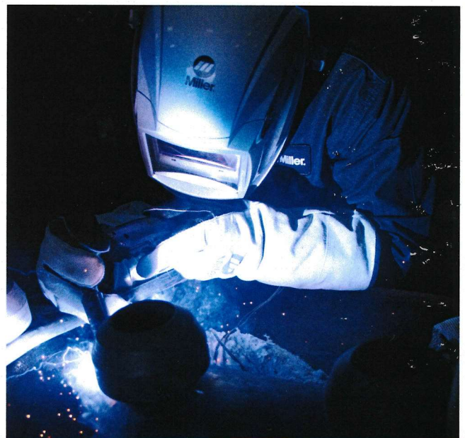
Once the TIG root is placed, welders switch to a gas-shielded Flux-Cored wire before eventually switching to sub-arc welding.
