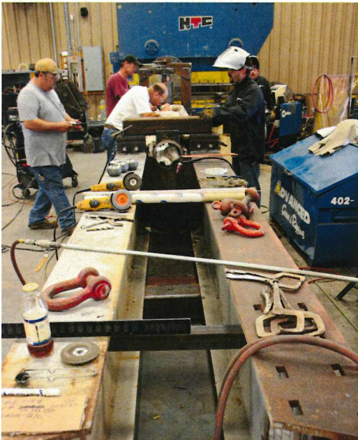
Topp's Mechanical has built custom jigs that allow for the header to be set right on top of the induction cables. This helps heat the piece from the bottom and minimize wrapping time.
